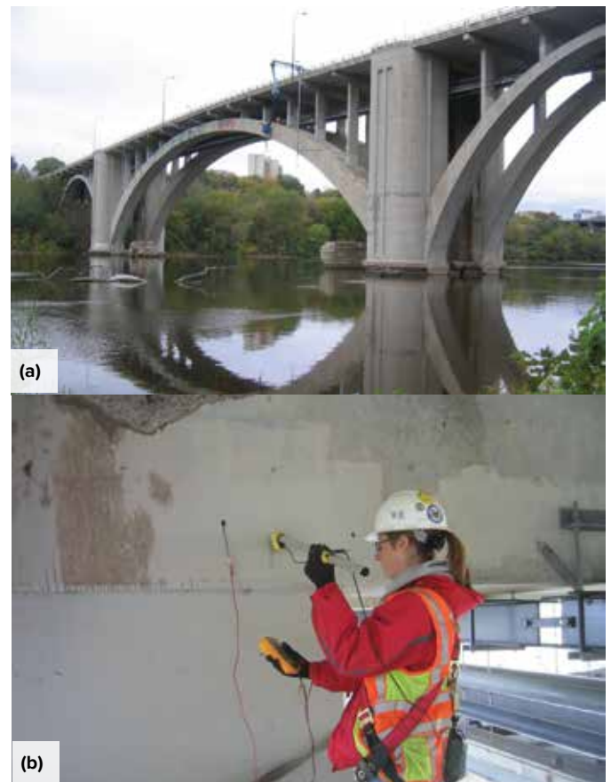
Fig. 2: Bridge investigation activities in 2007: (a) inspection, field testing, and material sample collection; and (b) half-cell corrosion potential measurements
