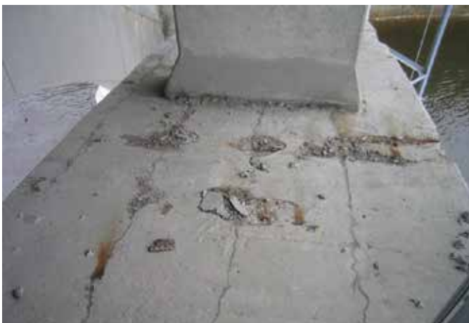
Fig. 5: Longitudinal cracking along interior lines of steel truss reinforcement
