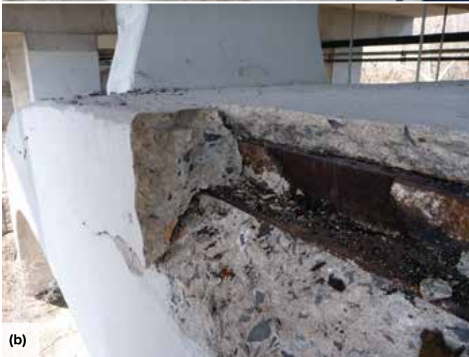
Fig. 4: Examples of arch rib distress conditions: (a) red arrows indicate cracking and delamination at corners, green arrows indicate cracking along interior lines of steel truss reinforcement, and blue arrows indicate freezing-and-thawing damage; and (b) loss of corner concrete caused by corrosion of steel angle
