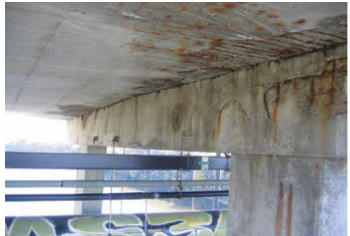
Fig. 6: Reinforcing steel corrosion and spalling due to leakage of expansion joint over cap beam
