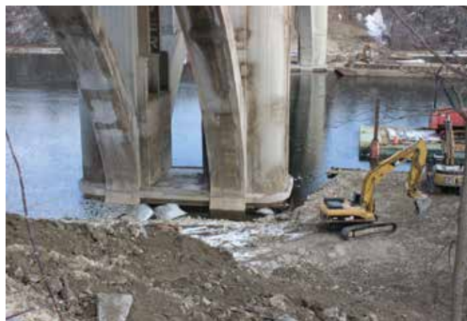
Fig. 12: Completed concrete jacket around base of river pier (after removal of coffer dam)
