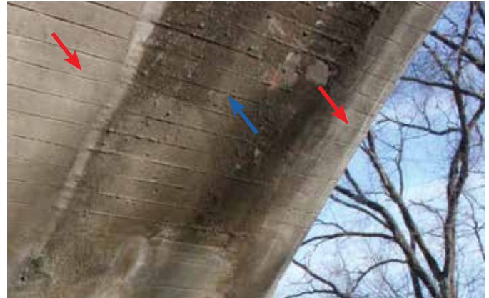
Fig. 9: Form-board finish on new repairs (red arrows) adjacent to original surface texture (blue arrow)
